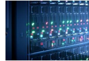
New Build Colocation Data Center Confidential Client | USA
